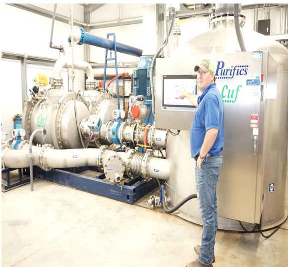
Figure 1: The CUF® System at Hilldale Water District, Vicksburg, Mississippi
