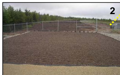
Recirculating Sand Filter
