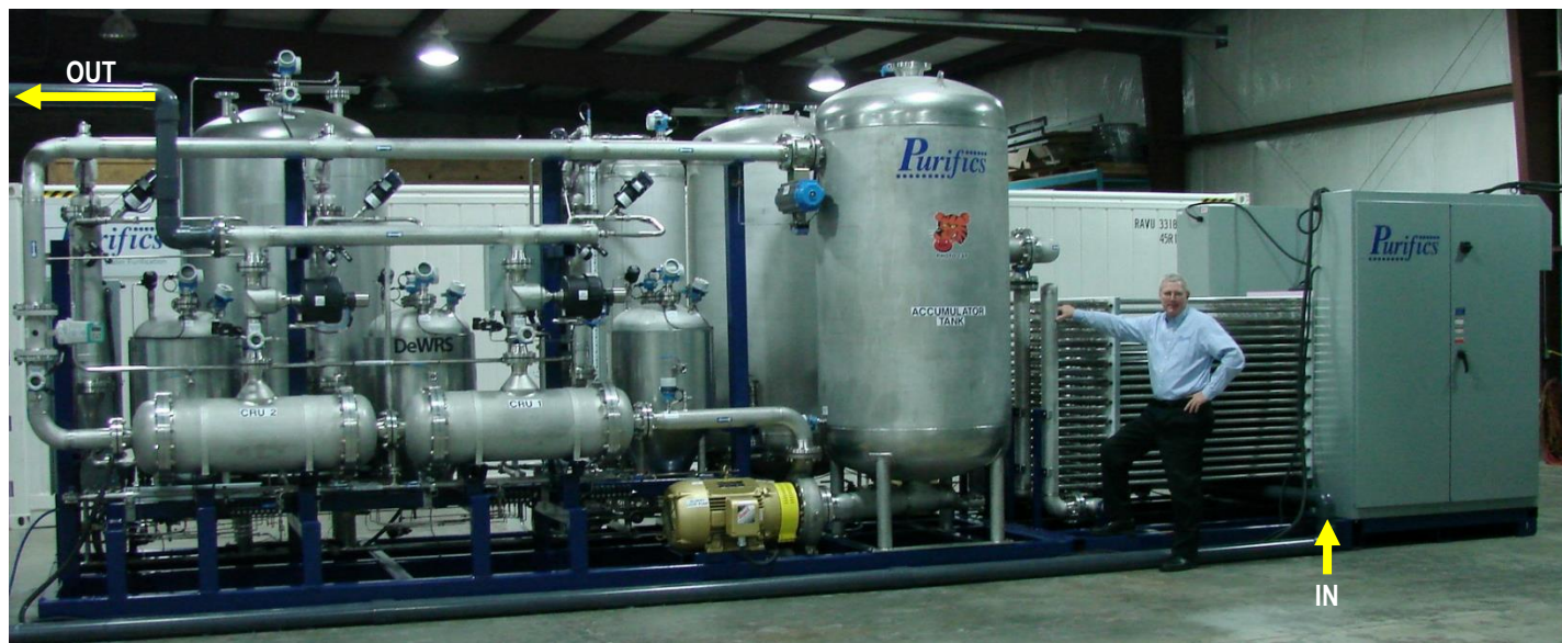
400gpm Photo-Cat Zero Liquid Waste, Hexavalent Chromium Reduction, Removal & Recovery
